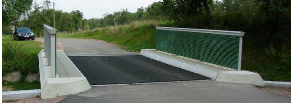
Klipphausen (Dresden), Germany. It is the first road bridge built from 100 % GFRP pultruded beams and deck, 2002
